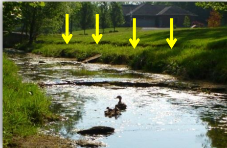
Tension crack bank failure along the entire length of the bank in the South Fork subwatershed at monitoring site SFG 5.3-UNT 0.1.
